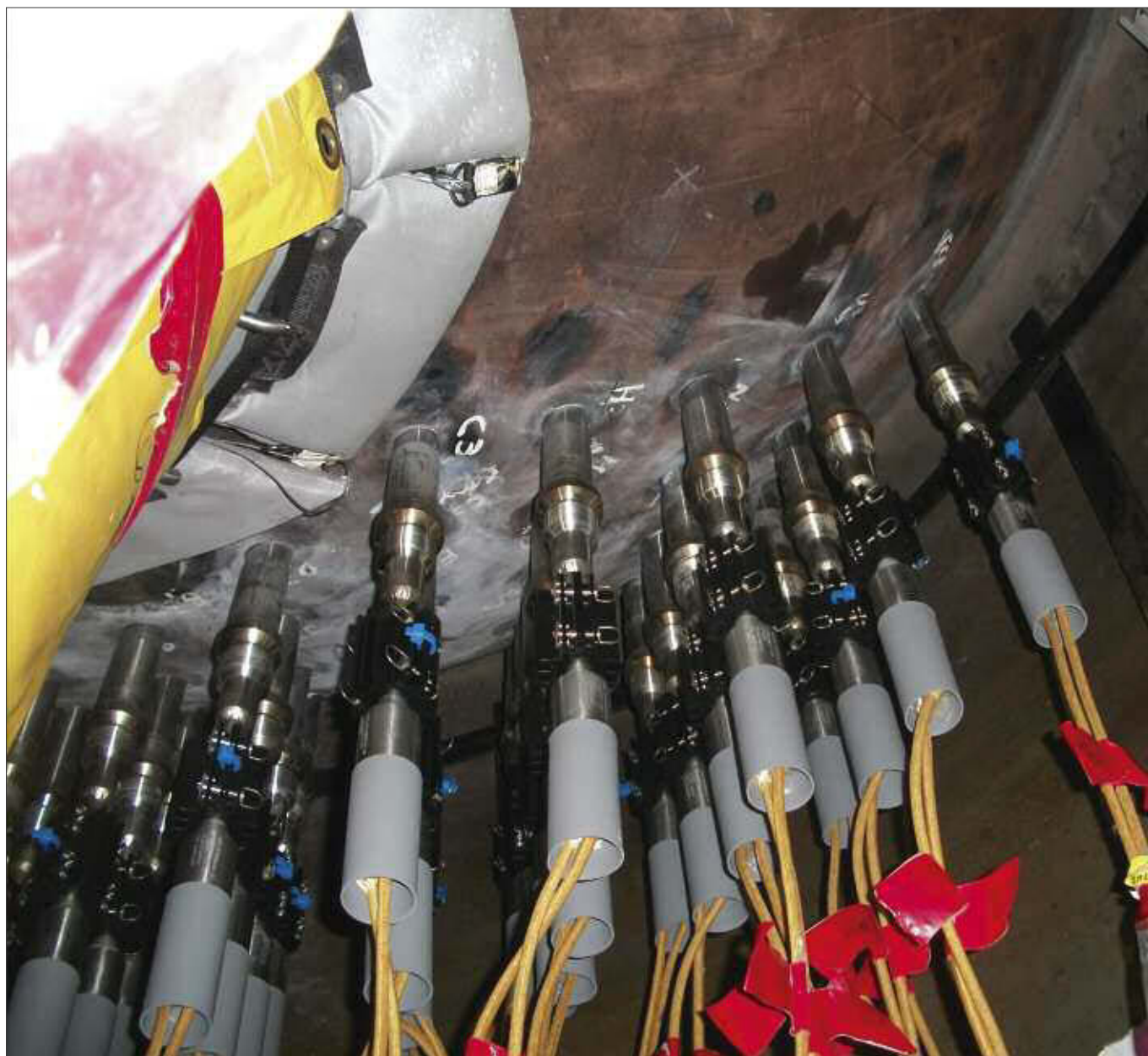
The final plant configuration with the new sleeves and heaters installed. The final electrical terminations have been made on the heaters.
