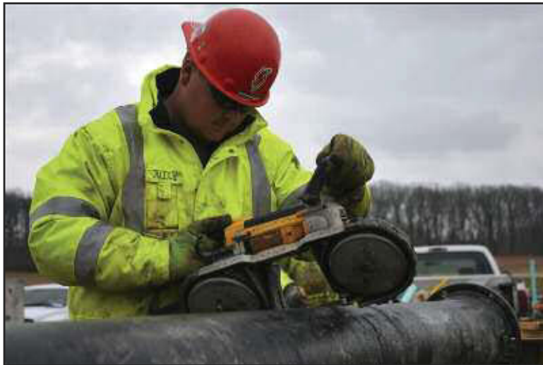
Justin Landrum, a Fluor-B&W Portsmouth employee, cuts a pipe during utility work installing new trailer complexes that will house personnel at the DOE Portsmouth site during the decontamination and decommissioning of the former gaseous diffusion plant.
