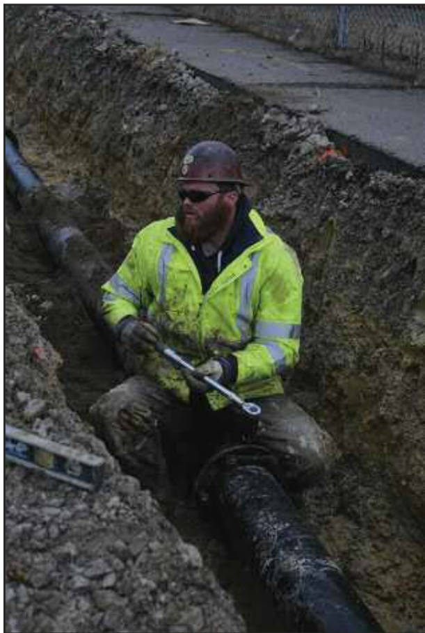
Fluor-B&W Portsmouth specialist Doug Martin works on the installation of utility lines in preparation for the installation of trailers that will provide office space as buildings are demolished.
