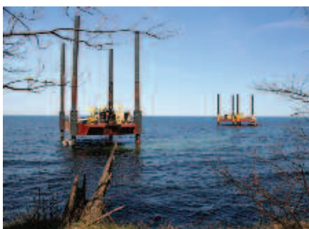
UniStar successfully completed boring 25 samples in Lake Ontario, which will be evaluated to determine the feasibility of constructing new cooling water intake tunnels for a potential third reactor at Nine Mile Point in New York.
