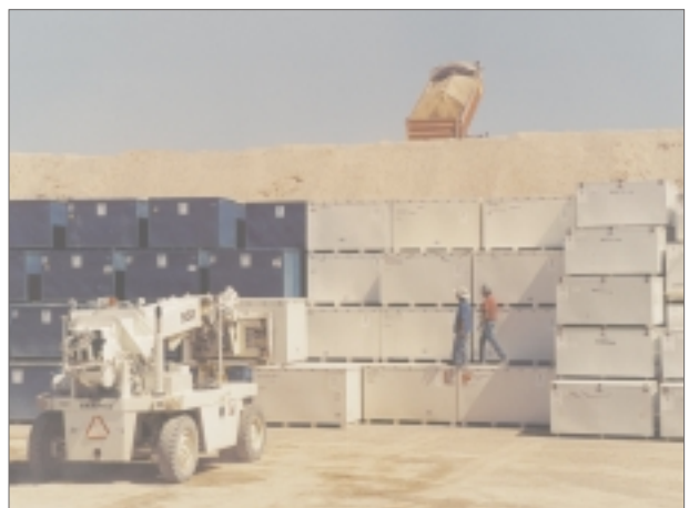
Waste disposal operations in Pit 5 of the Area 5 radioactive waste management site.
