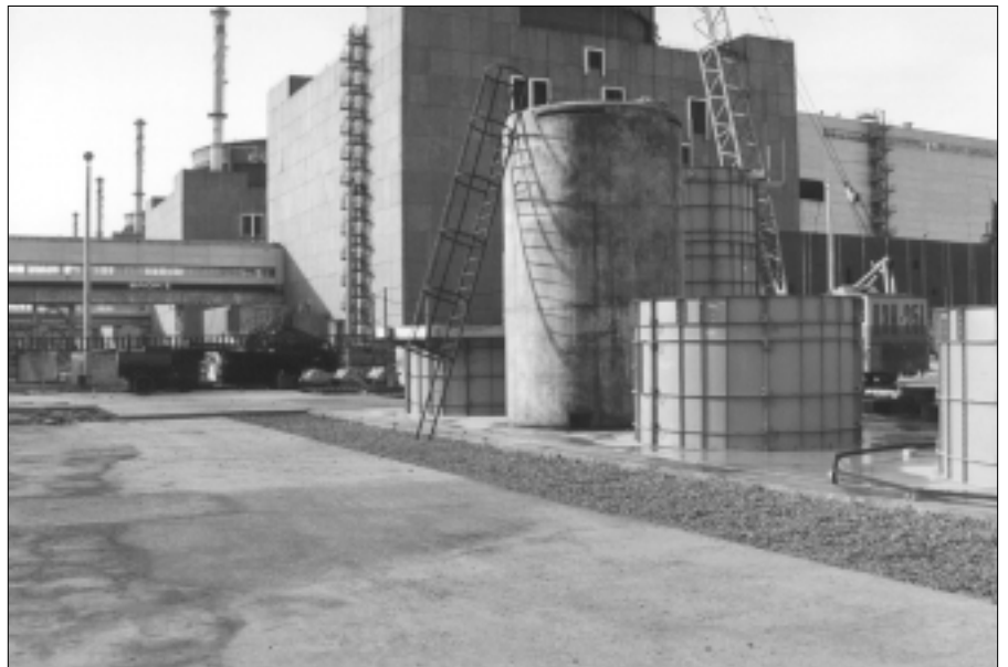
Forming the storage casks. The steel forms have been removed to reveal the concrete cask.
