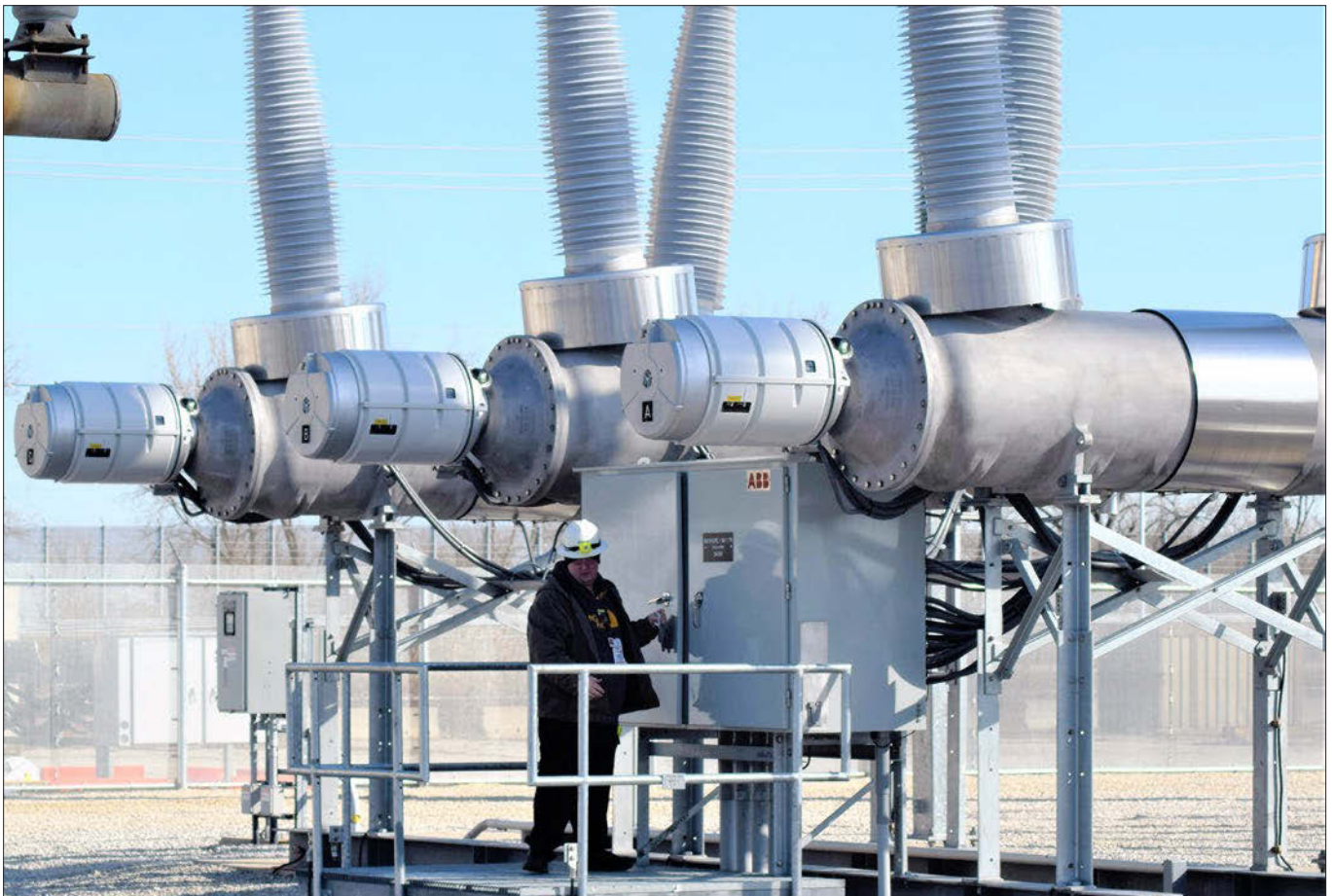
Operator Chris Simpson closes the control cabinet on the DB-34561 output breaker after switchyard work was completed.
