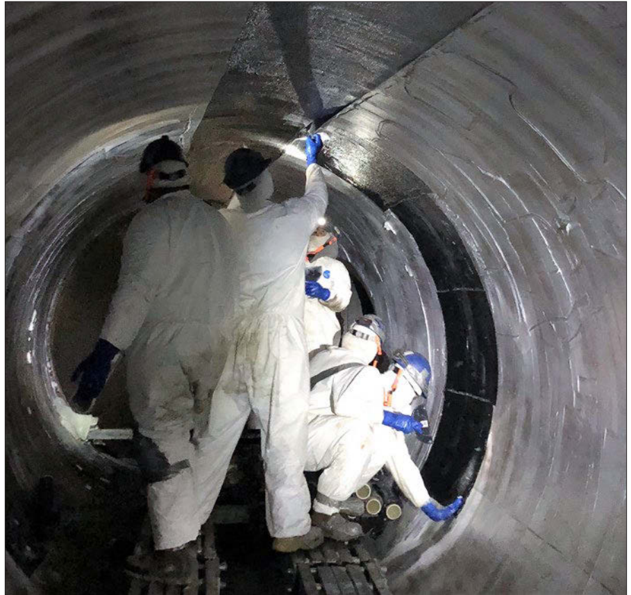
Technicians apply carbon fiber wrap to the inside of one of the two 108-inch circulating water pipes near the Davis-Besse cooling tower to help mitigate years of damage caused by falling snow and ice.
