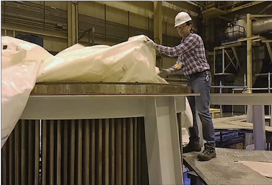
Project Manager Mark Wymer uncovers a tube bundle staged for replacement in one of the Davis-Besse condensate polishers.
