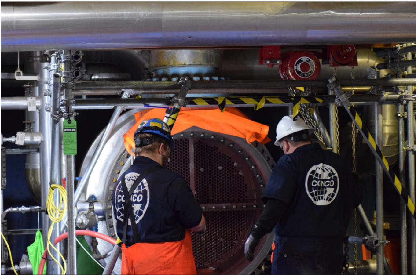
Workers prepare to reinstall the cover on one of the plant feedwater heaters during the outage.
