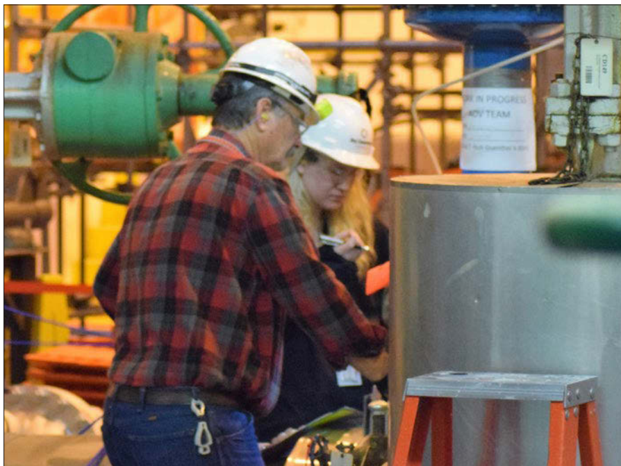
Members of the air-operated valve (AOV) maintenance team conduct work on a valve on the turbine deck. The AOV team conducted overhauls, calibrations, packing consolidations and adjustments, and diagnostic testing on 39 different valves during the outage.
