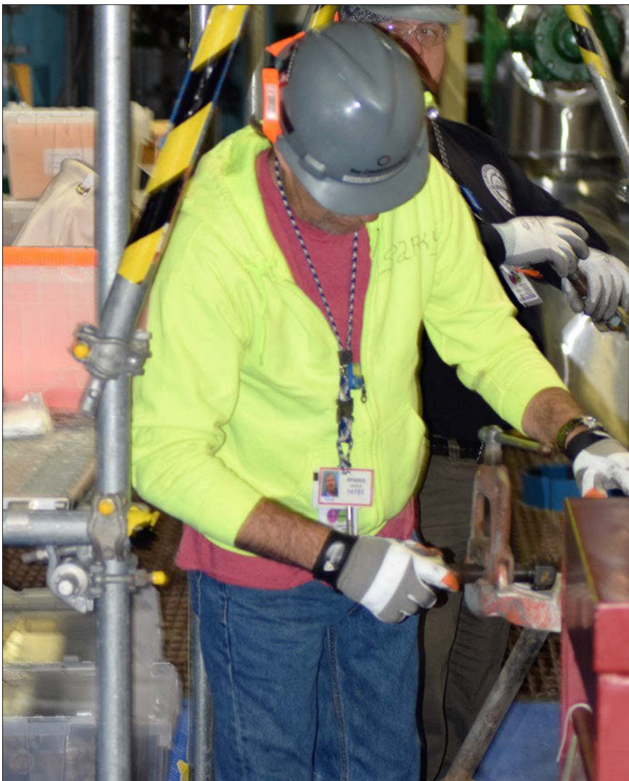
One activity not accounted for in the original outage scope was cleaning and refurbishing the bolts that hold the condensate polishers together. More than 400 bolts had to be blasted and cleaned, and any burrs or irregularities removed. Creative scheduling got this key task included in the outage work.
