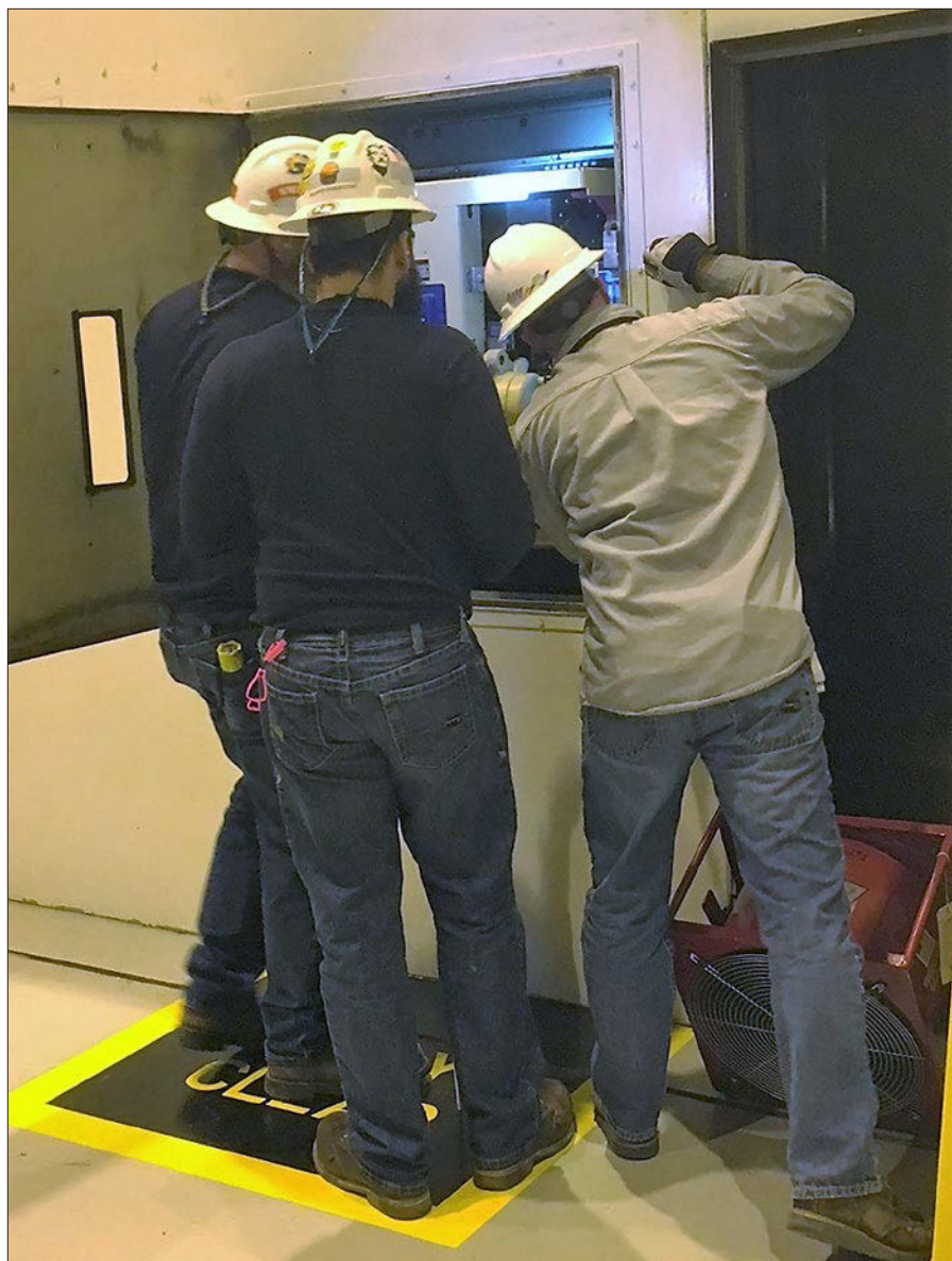
Plant electricians rack-in the exciter field breaker as Davis-Besse prepares to return to service following its IR20 outage.
