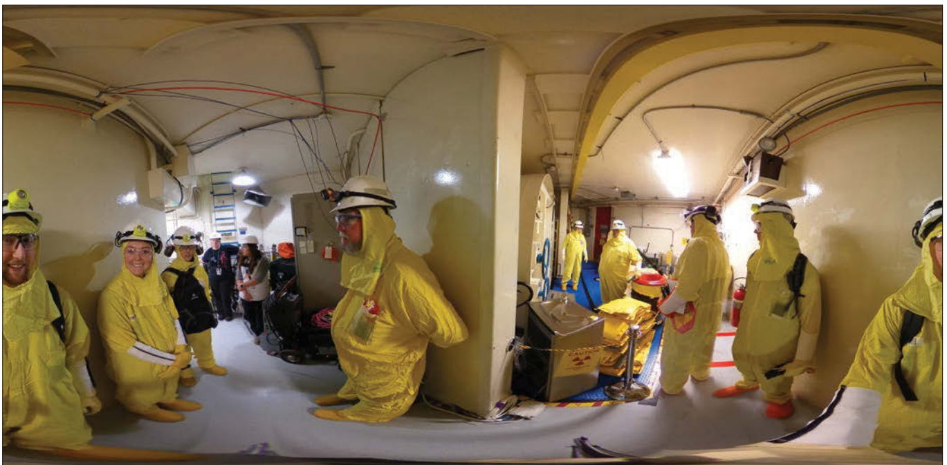
Crews wait outside the containment hatch to begin inspections at the start of the outage. A 360-degree camera with a fisheye lens was used to take the photo.
