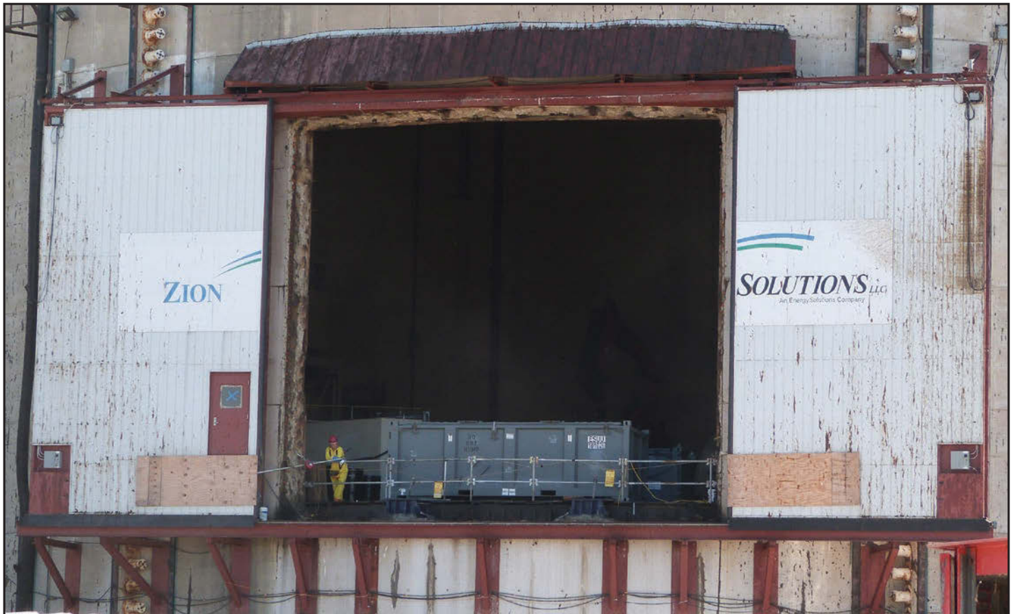
A worker stands in a doorway cut into Zion's Unit 1 containment building in July. ZionSolutions says it is on track to complete decommissioning by 2018.
