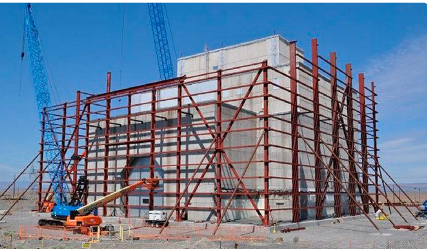
The first steel columns, each weighing up to 28 tons, were placed for a cocoon over the former K East Reactor building at the Hanford Site. (Photo: DOE-EM)
