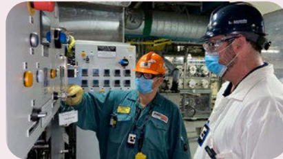
Workers examine the He-3 extraction tool at Darlington. (Photo: Laurentis)
