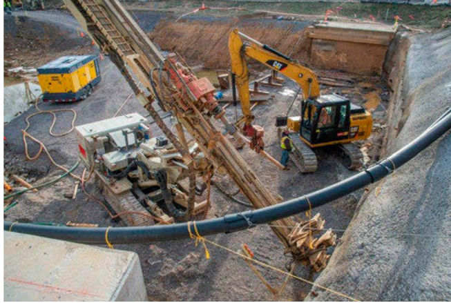
Crews at the headworks site of the Outfall 200 Mercury Treatment Facility excavating for the construction of foundations.
