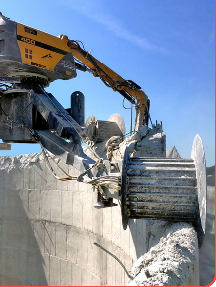
Above: An example of the MANTIS system being used at a stack demolition project outside of Brookhaven. (Photo: ICC Commonwealth)
