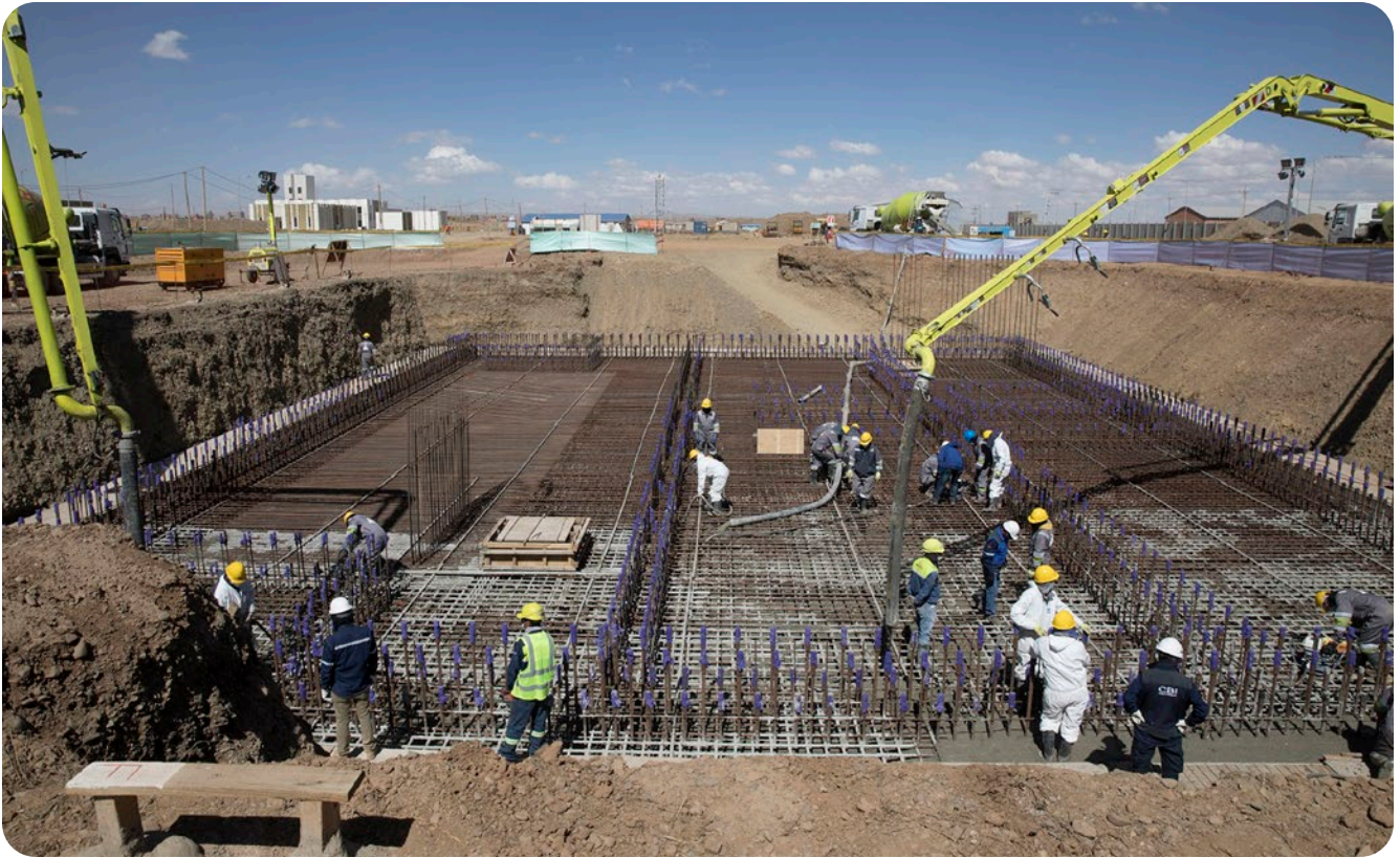
First concrete pour for the research reactor begins at a Bolivian nuclear research center. (Photo: Rosatom)
