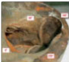
Advanced Boric Corrosion
