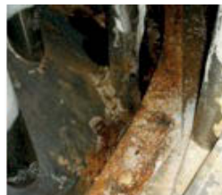
Boric acid Corrosion of Lid
