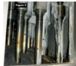
Boric acid deposits from Leak on Pen. #77
