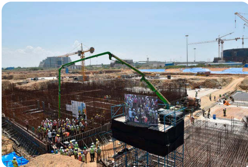
India’s Kudankulam plant, during the June 29 Unit 5 construction launch ceremony. (Photo: Rosatom)
