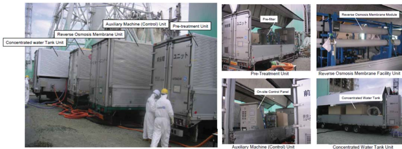
Figure 12. Photographs of portable water cleanup and decontamination treatment units. (Courtesy of TEPCO.)
