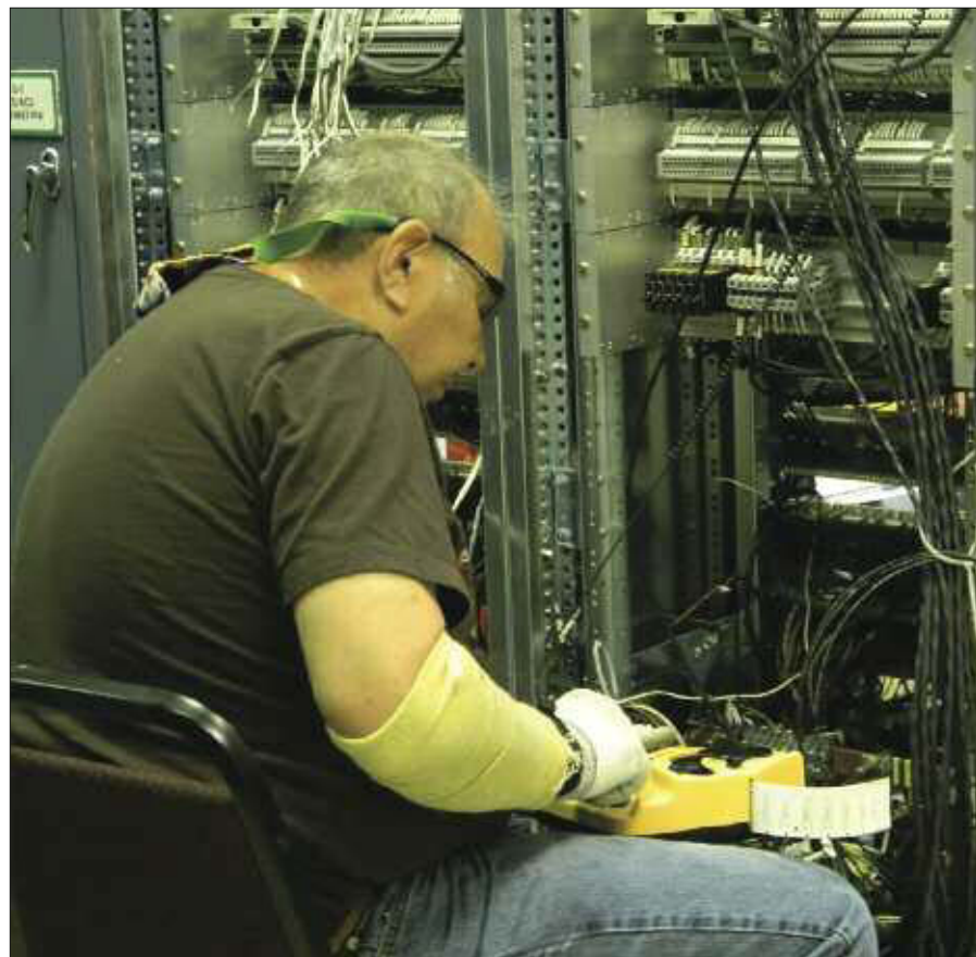
The upgrade to digital I&C at Oconee-1 involved extensive disconnection from the original analog equipment and reconnection to equipment in new cabinets.
