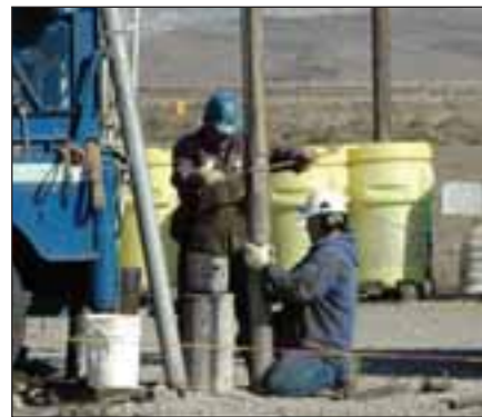
Well drilling at Hanford. The article beginning on page 26 looks at work being done on the vast site's Central Plateau.
