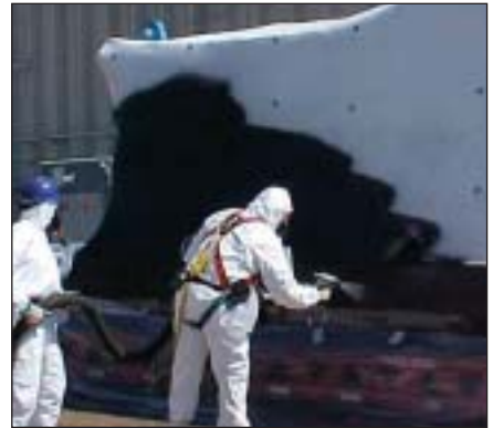
Graffiti at a work site? No, workers creating a cover for a large chunk of waste. See article beginning on page 40 for more on this technology.
