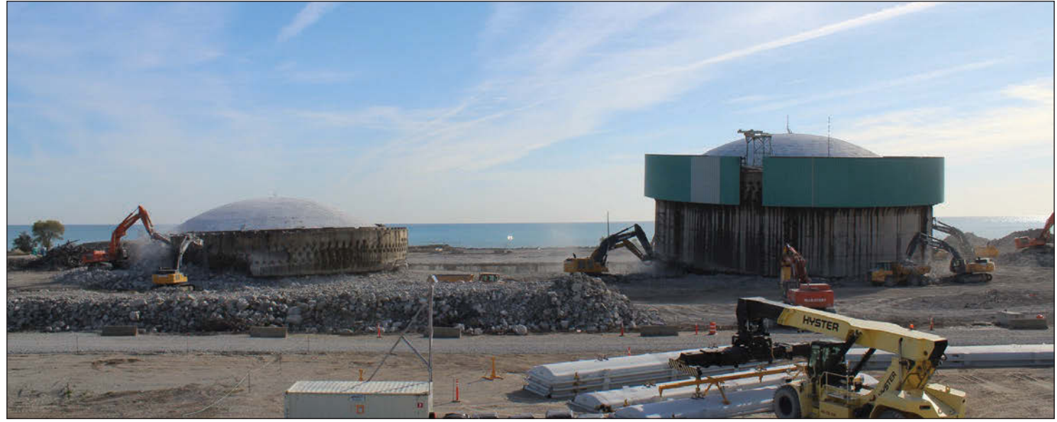
The Zion Station decommissioning project in Illinois was the first-of-its-kind, license stewardship agreement for the decommissioning, site restoration, and dry fuel storage of a U.S. commercial nuclear power plant. EnergySolutions completed major D&D work ahead of schedule.
