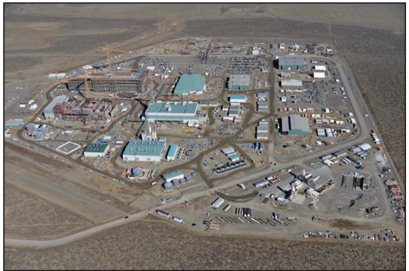
Technical issues have delayed the completion of Hanford's Waste Treatment and Immobilization Plant, known as the Vit Plant. (Photo: DOE/BNI)
