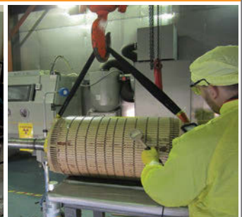
In-House Decon Facility
