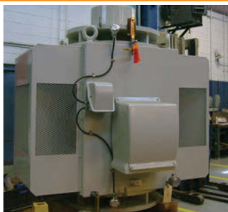
Safety-Related Motor Repair
